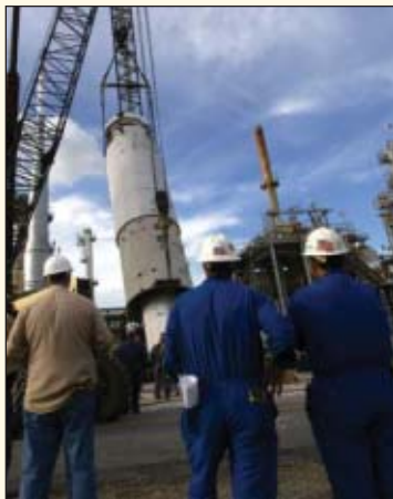
Workers oversee the day-long process of installing Placid Refining Co.'s new FCC reactor at its Port Allen, La., refinery. Photo from Placid.
